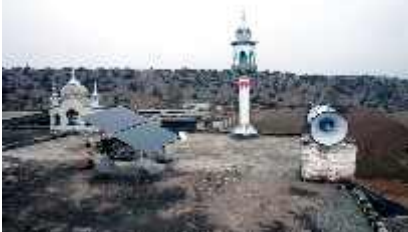
Solar panel installed on the roof of the mosque
